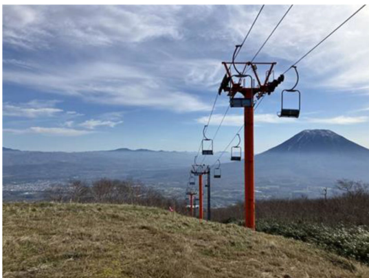
Ace Lift #3 (existing lift)
